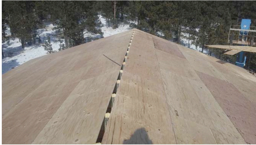
Leave an Opening or Slit the Ridge if Using Roof Ridge Vents. Better to not let a roofing contractor do this step.
