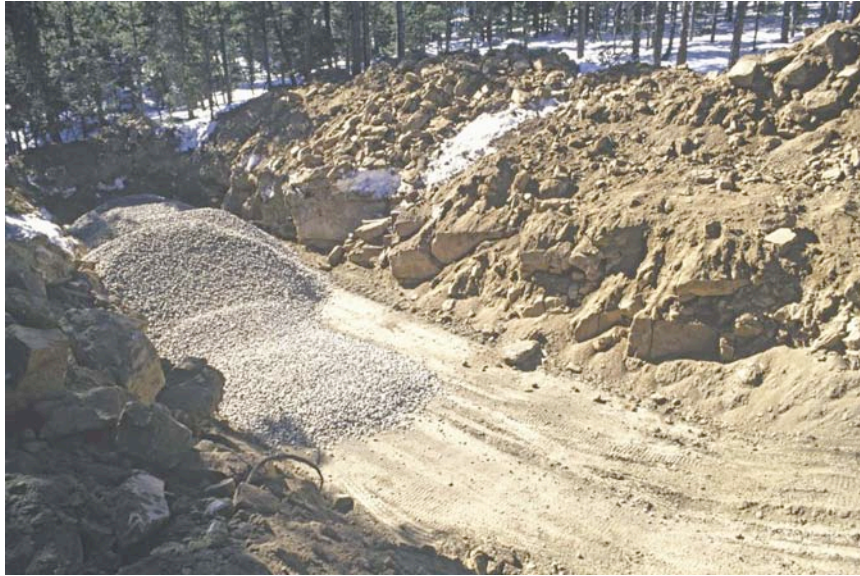
A Leech Field is Needed with a Septic Tank to Minimize Septic Pumping.
