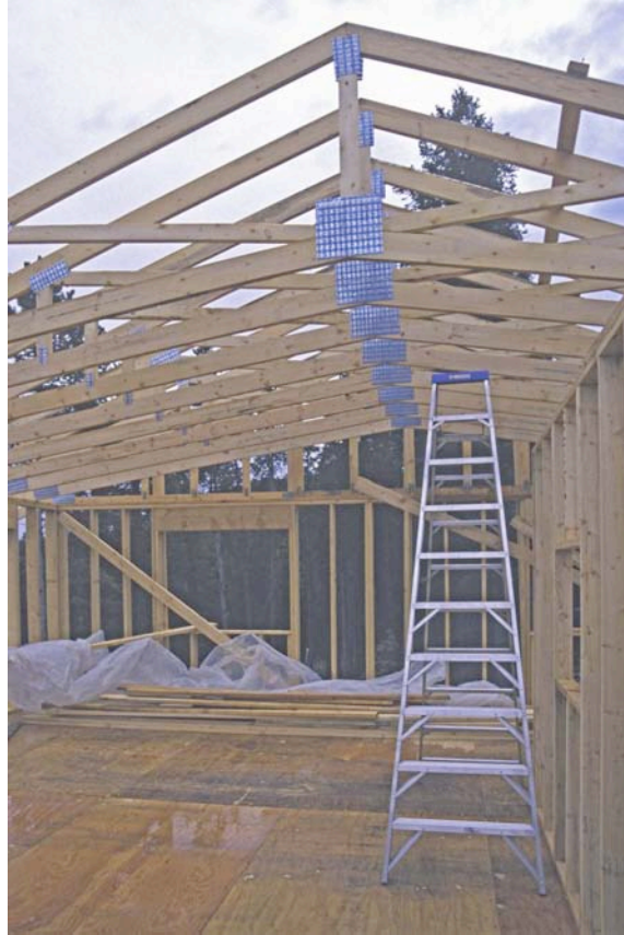
A 10 ft Step Ladder is Needed for Vaulted Ceilings to Reach Roof Trusses and Secure Them with a Temporary 2x4. Note that the thick plywood floor is wet with recent rainfall. If it was an OSB floor, it would be warped with the rain.
