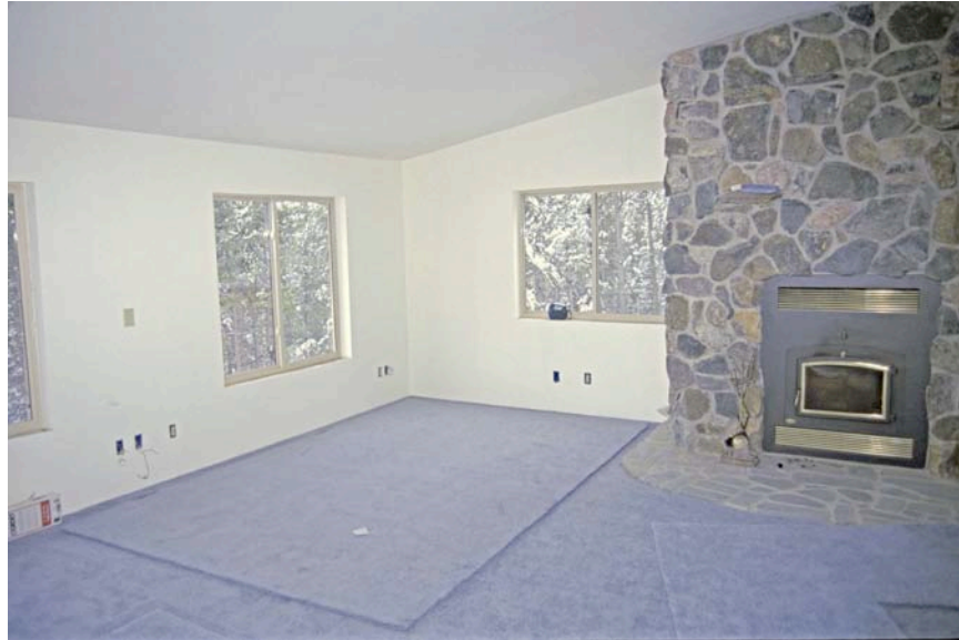
Carpet in the Process of Installation after Painting and Floor Tile is Completed
