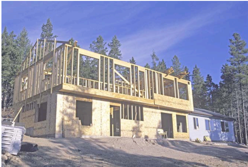
Installing the Gable Truss Now it is easy for one person to slide the trusses to the other end and rotate them up. A special slanted platform ladder helps to rotate them up.
