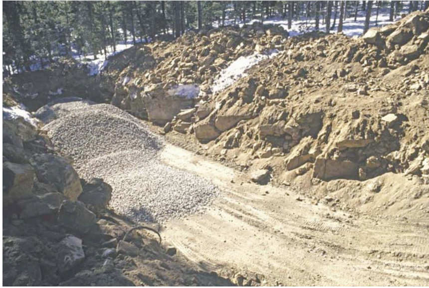
A Leech Field is Needed with a Septic Tank to Minimize Septic Pumping.
