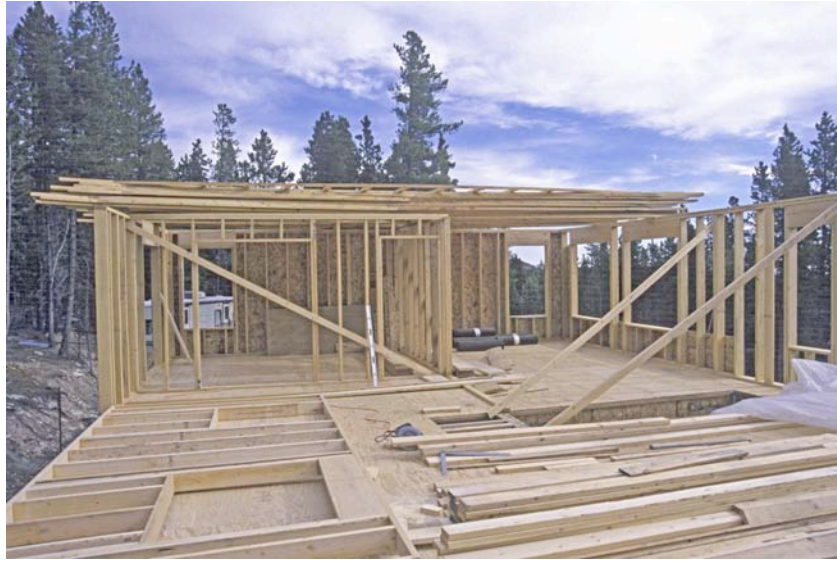
Roof Trusses Stacked in Order and More Walls Ready to Be Lifted. It is easy for two tall people to lift the trusses on the 2 nd floor framing before installing all the framing. Otherwise you'll have to rent an expensive crane.
