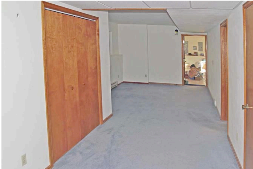
HVAC Ductwork is Hidden in the False Ceiling and Boxing Overhead
