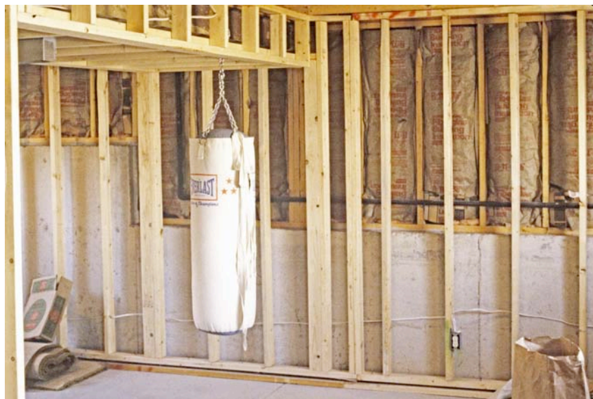
A Steel I-beam (just above the punching bag that is difficult to see) at my 1 st Home.
